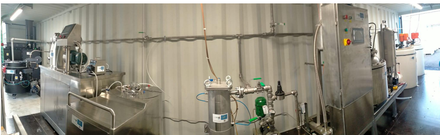
Pilot plant overview
